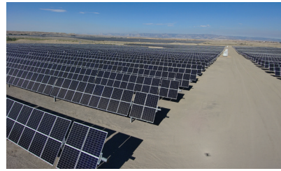
GRAPHITE SOLAR I 104MW Solar Facility in Wellington, UT.
