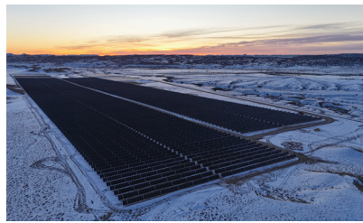
RPLUS ENERGIES GREEN RIVER ENERGY CENTER A 540MWdc PV plant and associated 400MW/1600MWh battery storage facility on over 2,500 acres of previously undeveloped high-desert land in Emery County, UT. Work included installation of 125,000 piles and nearly 1,000,000 PV modules. One of the largest PV facilities in the state.
