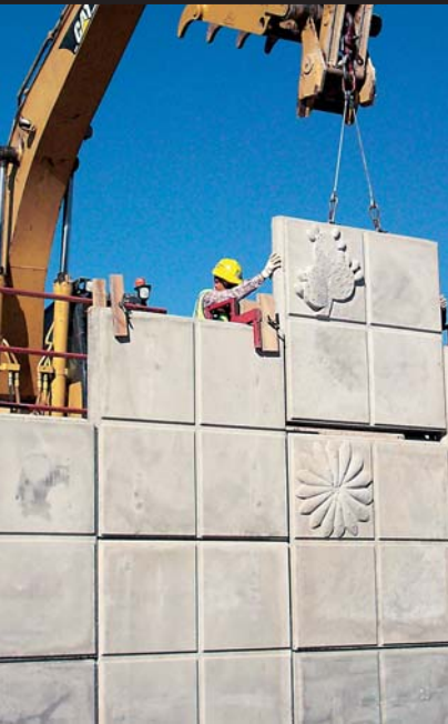
Below: Crews install abutment wall panels featuring some of the project's extensive architectural concrete details.
